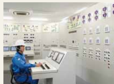
Centralized control room
